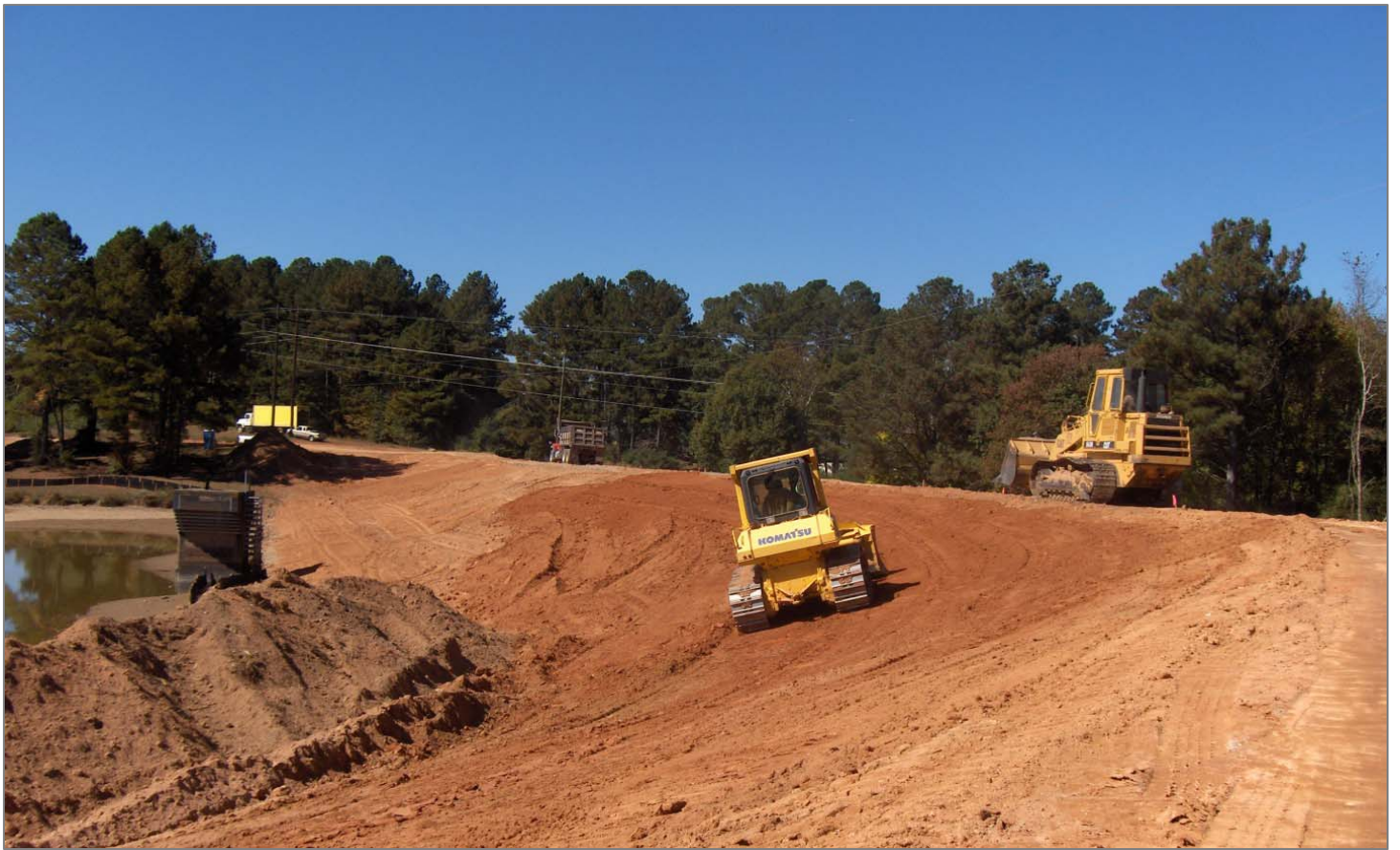
J&K Utilities brings in fill dirt and re-grades the slope of the dam.
