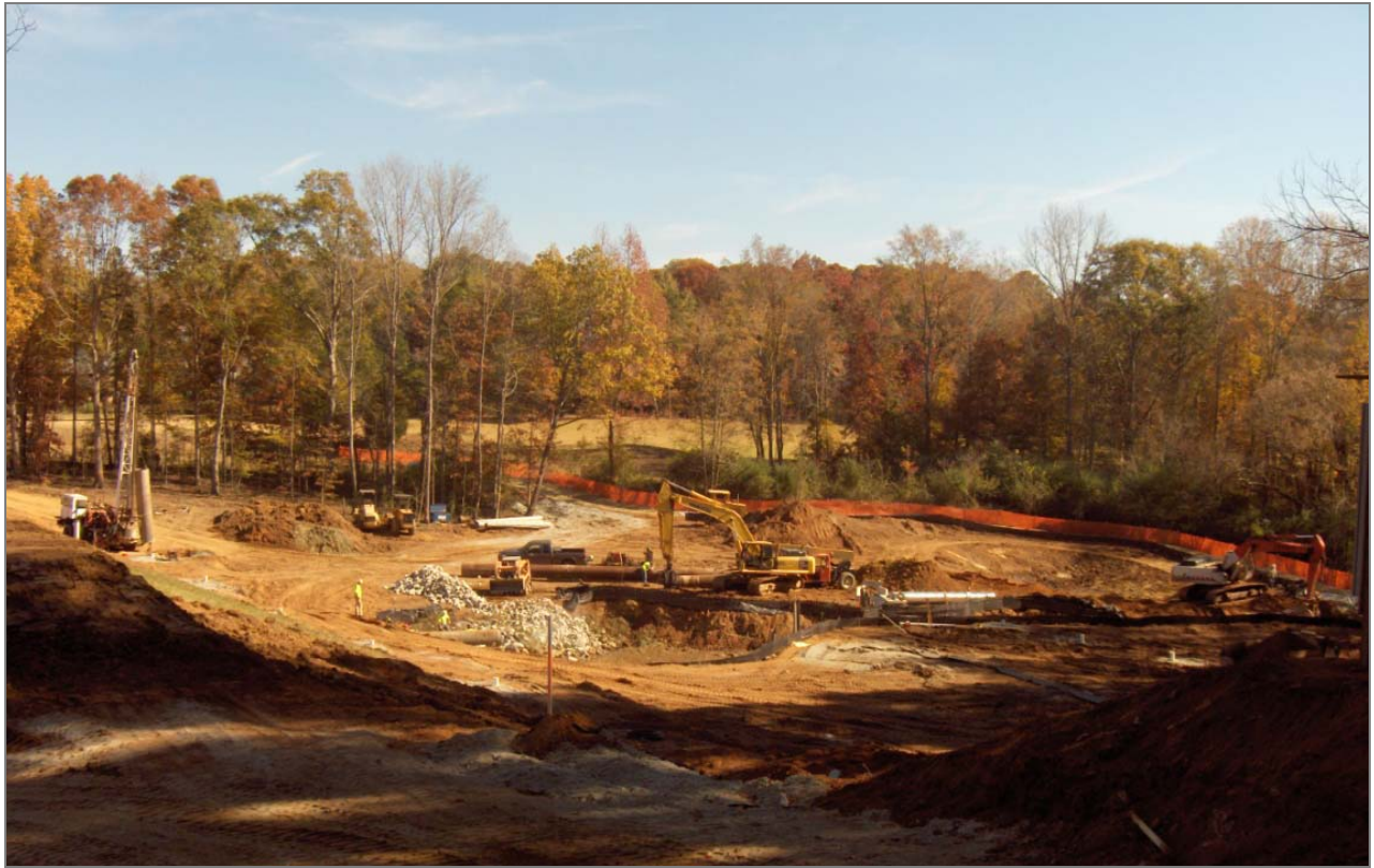
The crew begins regrading the back slope of the dam and excavating the site of the new spillway.
