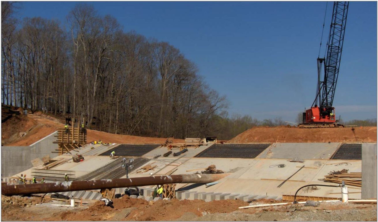
March 2011 - A view of the concrete spillway from the backside of the dam
