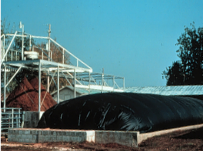
An operational anaerobic digester
