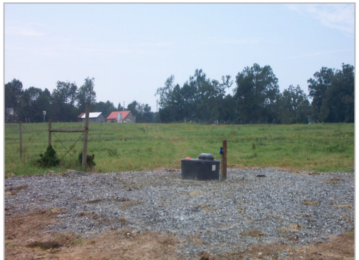
Heavy Use Area improvements include a new watering tank and gravel to protect the area
