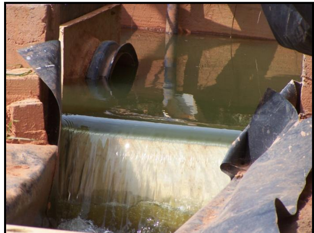
Figure 18. Flow into Channel at Weir
