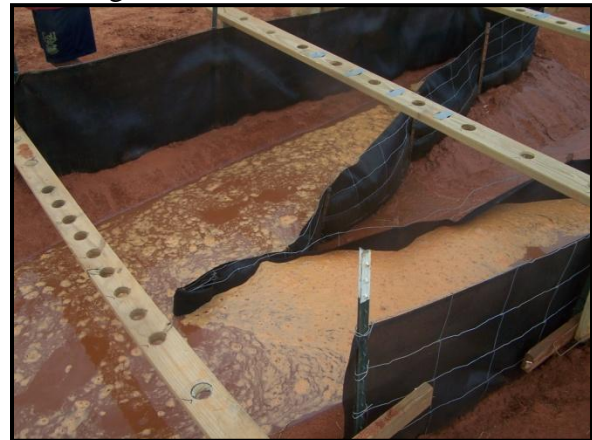
Figure 24. Silt Fence Check Structure
